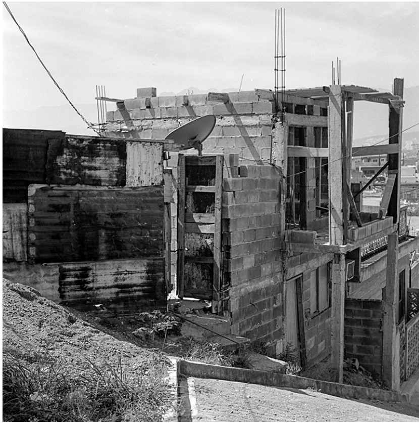
Figure 4: The region's self-built architecture mainly uses materials extracted from the quarries. Colonia Tierra y Libertad, Cerro del Topo Chico, 2019.
