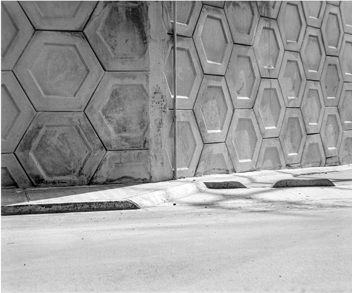
Figure 3: Concrete bridge, near sand-selling businesses in the Cerro del Topo Chico area, 2019.
