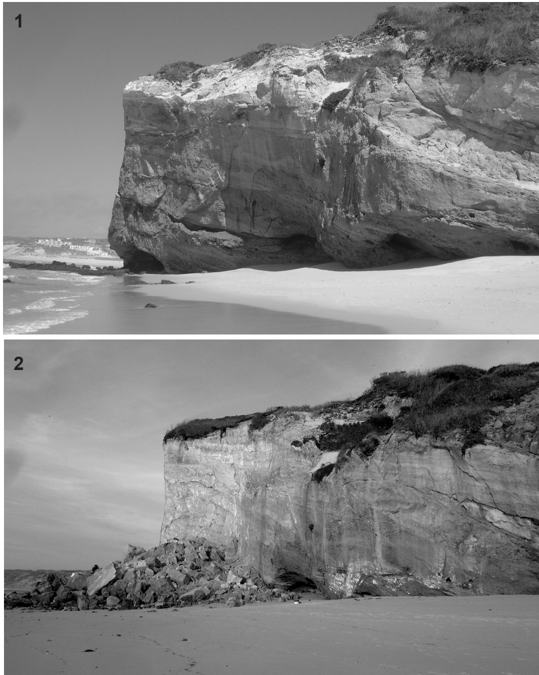
Fig. 12.- April, 1 2004 rockfall. 1 -cliff before the rockfall event; remark the well developed notches at the cliff base; 2 -cliff after the rockfall event (Photo 1 -August 2003; Photo 2 - April, 2004).
