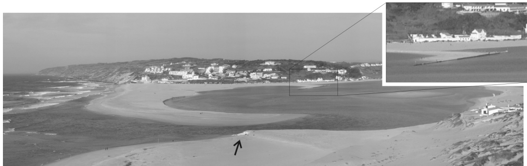
Fig. 14.- The groyne constructed in the Obidos lagoon near its northern margin. The arrow points to the location of the sand bags placed to reduce south dune erosion.
