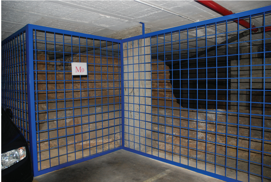
Figure 9. Earth Countermines from the Front from the 18 th century. Located in the property's car park and protected by a grate. Calle Tamarindos, Cádiz. Lara Delgado Anés.
