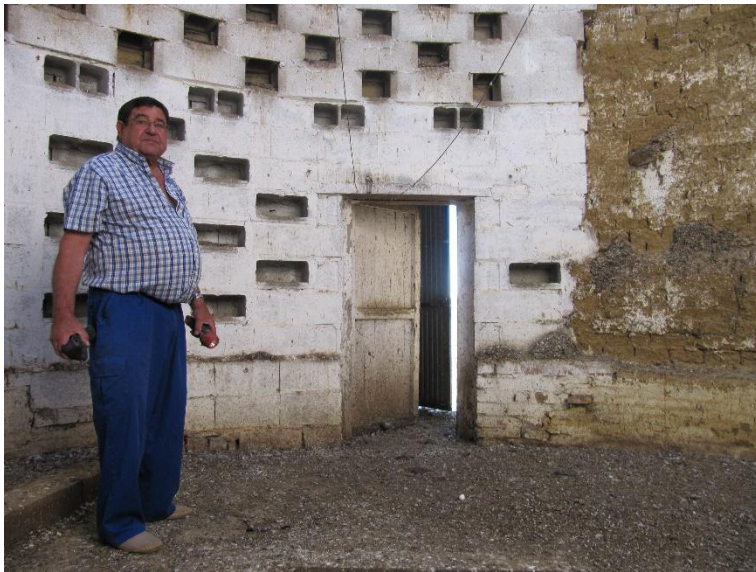
Fig. 2. Dovecote in Pozuelos del Rey (Palencia, Spain). The modern adaptation of a historical vernacular building represents an authentic expression of the present-day culture of the area. The modernisation was made by the building’s owner and to make the dovecote functional rather than simply picturesque. Photographed by the author.
