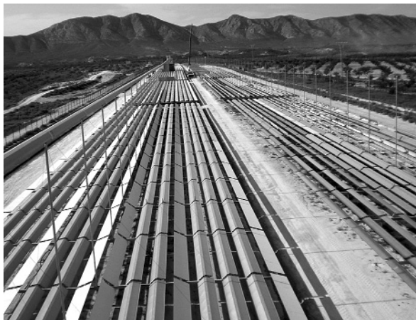
Figura 8. Central Puerto Errado 1
